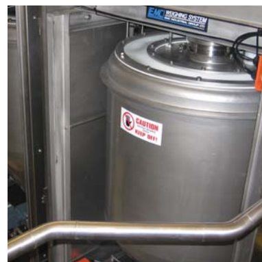
EMC Loss-in-Weight Salting System
